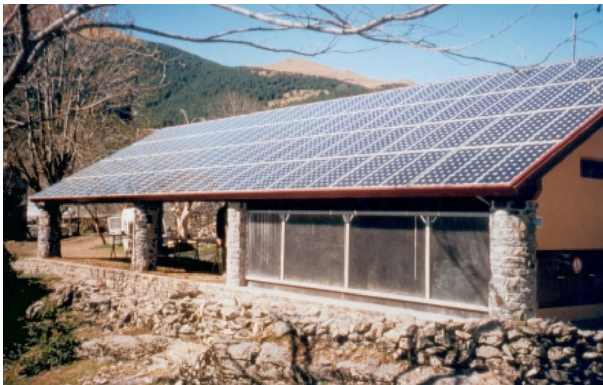
Figure 2: Centralized DC-bus system: electrification of the village of Escuaín (Huesca, Spain)
