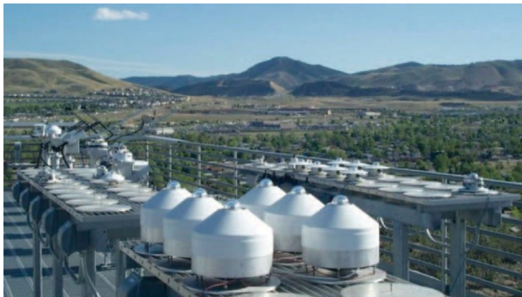
Figure 3-10. Kipp & Zonen model CM22 pyranometers installed in CV2 ventilators. Photo from NREL
