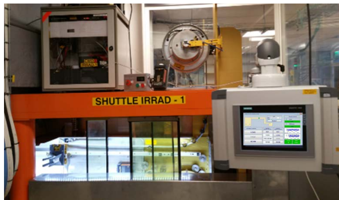
Fig. 5. LOAD position of the shuttle IRRAD1, outside the control room of IRRAD. The users' interface depicted in Fig. 6 is also visible here.
